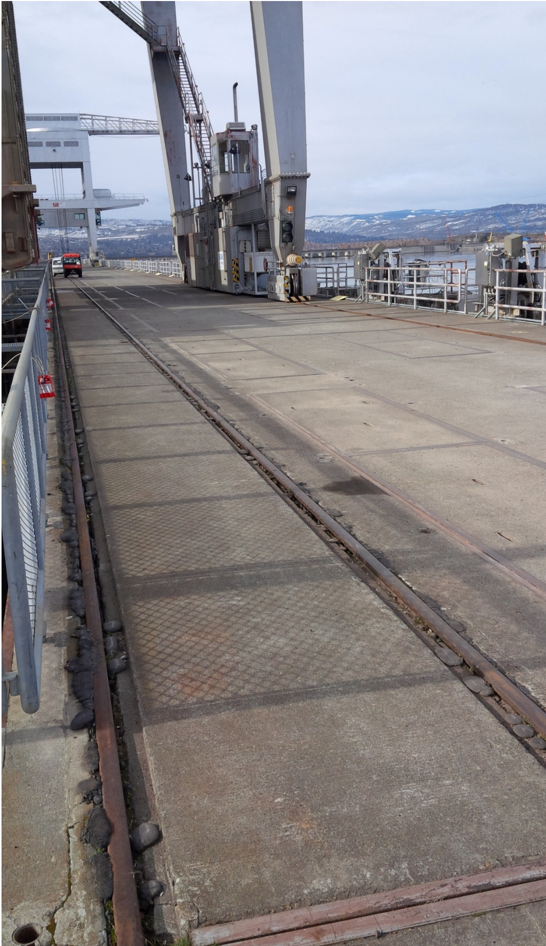
Derelict rail at unit 18 forebay deck. Unit 18 sluiceway gearboxes in background.
